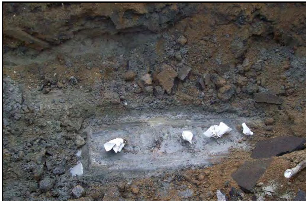
PHOTOGRAPH 2: 550-GALLON UST ENCOUNTERED WITHIN TEST PIT #1. THE UST WAS IDENTIFIED TO HAVE BEEN CLOSED IN PLACE AND FILLED WITH CONCRETE.
