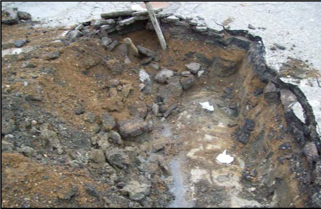
PHOTOGRAPH 5: 550-GALLON UST ENCOUNTERED WITHIN TEST PIT #2. THE UST WAS IDENTIFIED TO HAVE BEEN CLOSED IN PLACE AND FILLED WITH SAND.
