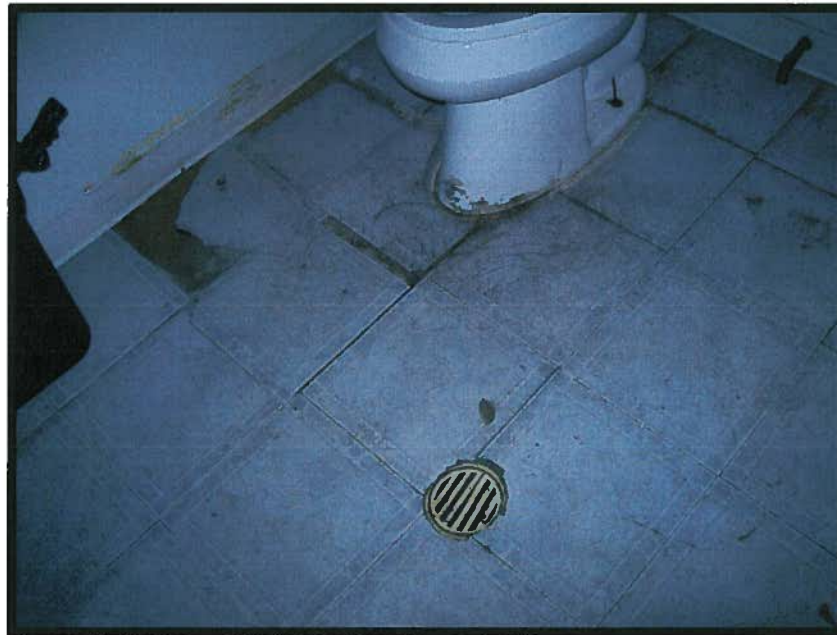
PHOTOGRAPH 6: SUBJECT PROPERTY VIEW OF A FLOOR DRAIN IN THE RESTROOM OF THE SUBJECT BUILDING
