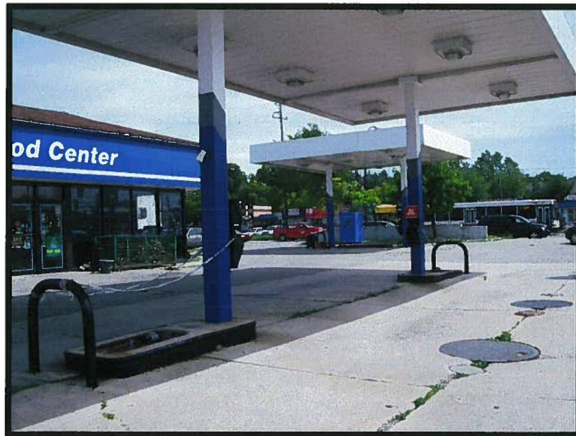
PHOTOGRAPH 10: SUBJECT PROPERTY VIEW OF OUT-OF-SERVICE DISPENSER ISLANDS LOCATED IN THE WESTERN AND SOUTHERN PORTIONS OF THE SUBJECT PROPERTY
