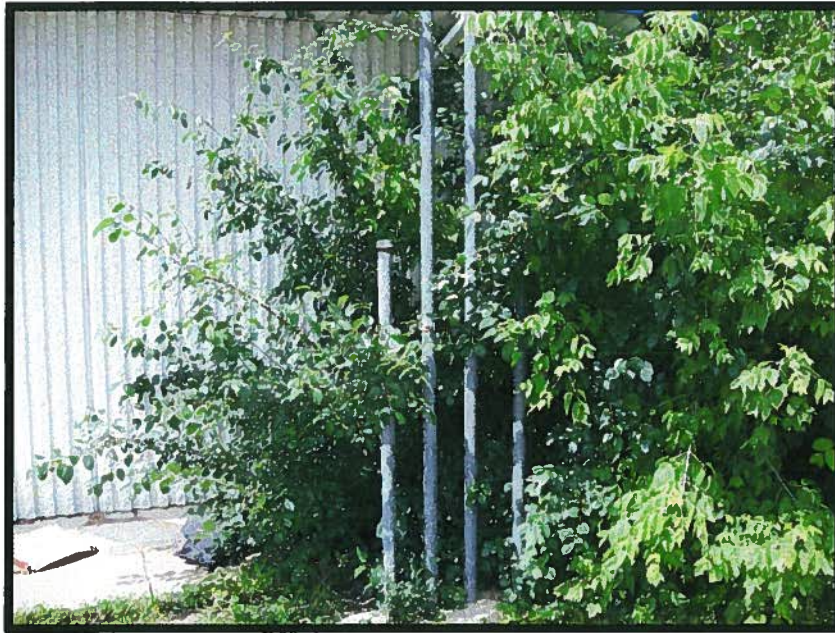
PHOTOGRAPH 7: SUBJECT PROPERTY VIEW OF TWO VENT PIPES ALONG THE SOUTHEASTERN WALL OF THE SUBJECT BUILDING
