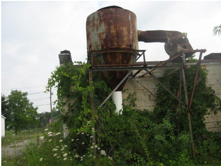
PHOTO NO. 6: Dust collection system at southwest corner of manufacturing building.
