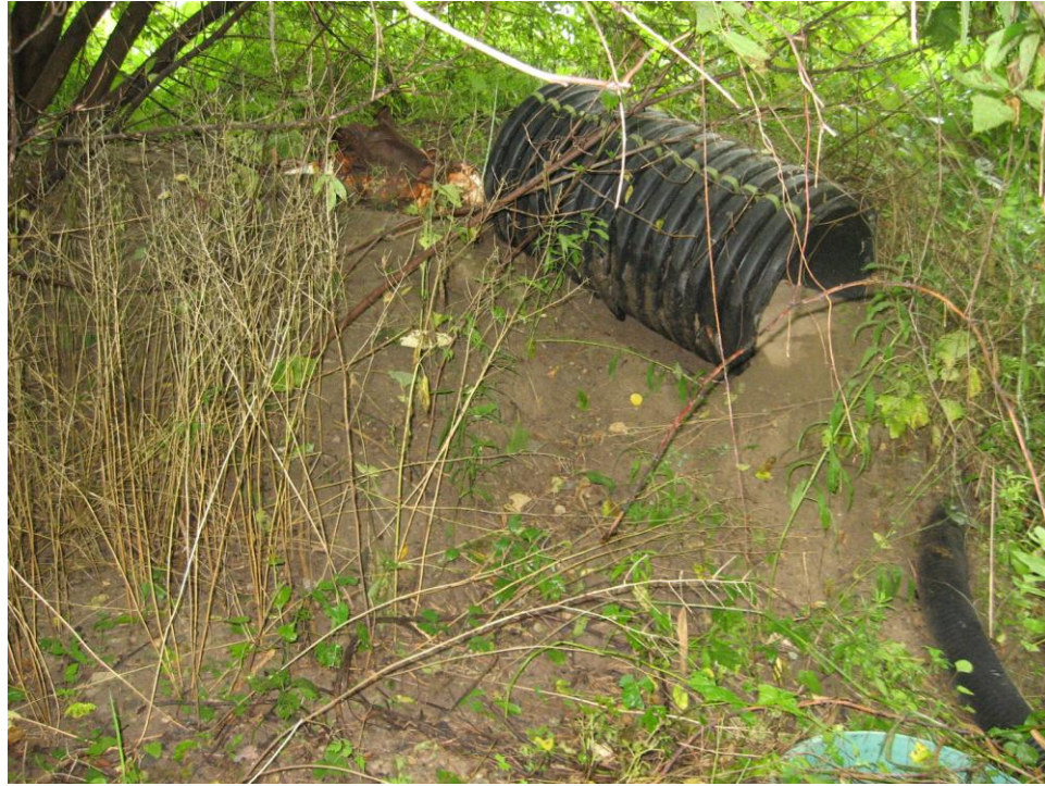
PHOTO NO. 13: Debris in creek bed along south Property boundary.
