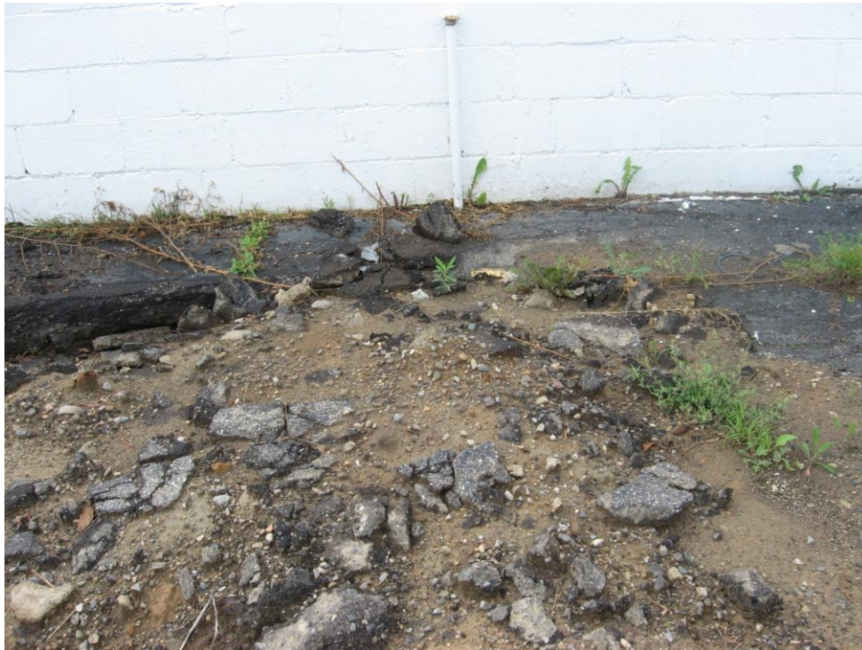
PHOTO NO. 4: Vent pipe and broken black top at north side of manufacturing.
